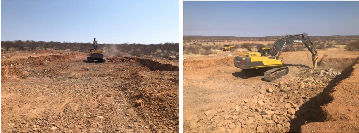
Figure 3: "Free-digging" - soft material is excavated to 1.5 m (left) and an additional 0.5-1 m is removed after mechanical rock breaking (right)
